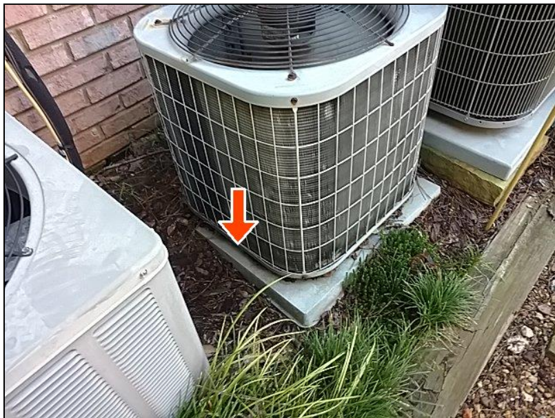
2nd floor condenser
