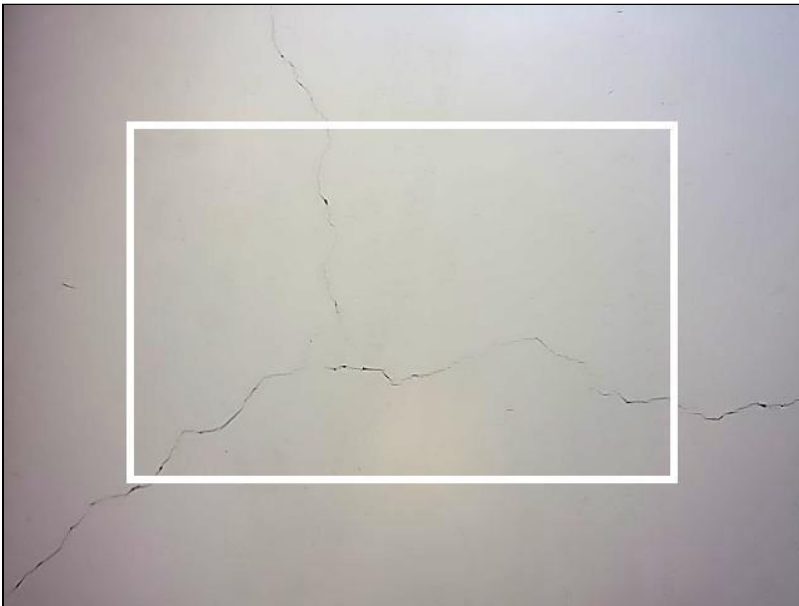
This location: Left
