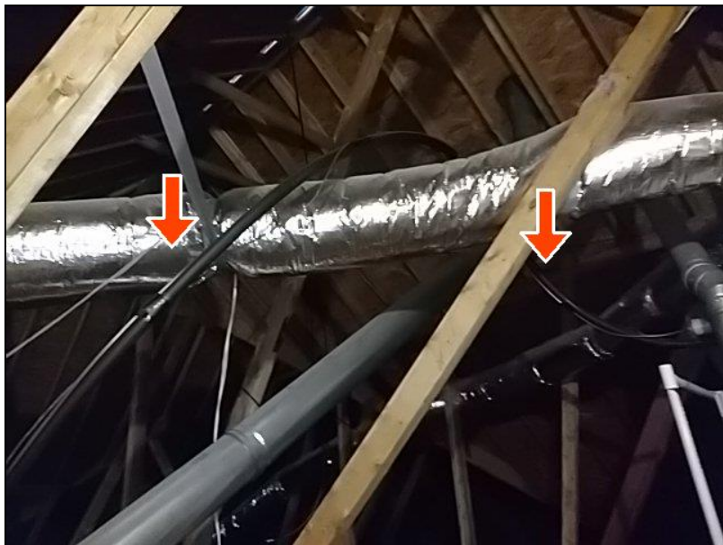
2nd floor line set
